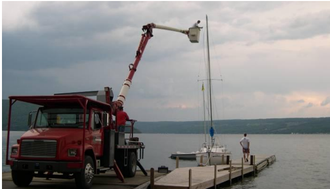
Brien Gardener gets a lift to repair his mast (Wednesday, July 16 th )
